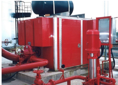
ITT A-C UL/FM Fire Pump with Acoustic Enclosure
