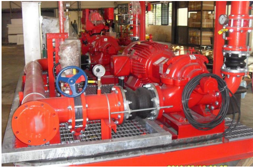
Skid Mounted ITT A-C UL/FM Fire Pump Package
