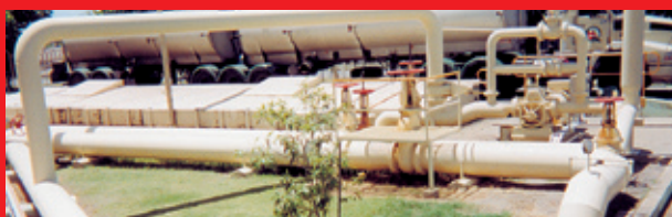
Molasses unloading facilities
