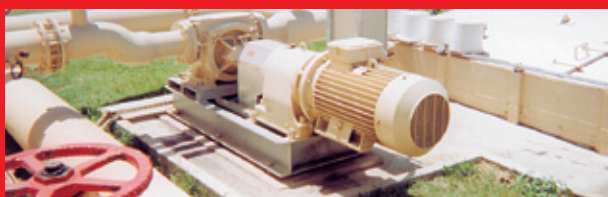
Sugar Terminal Installation
